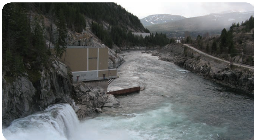
The sheet pile wall, constructed in 2008 to divert flows from the Brilliant dam away from the Brilliant Expansion tailrace, is visible in this photo taken from the roadway across the Brilliant dam.
