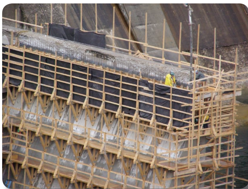
A close-up view of the concrete rehabilitation work at the Brilliant dam, spring 2010.
