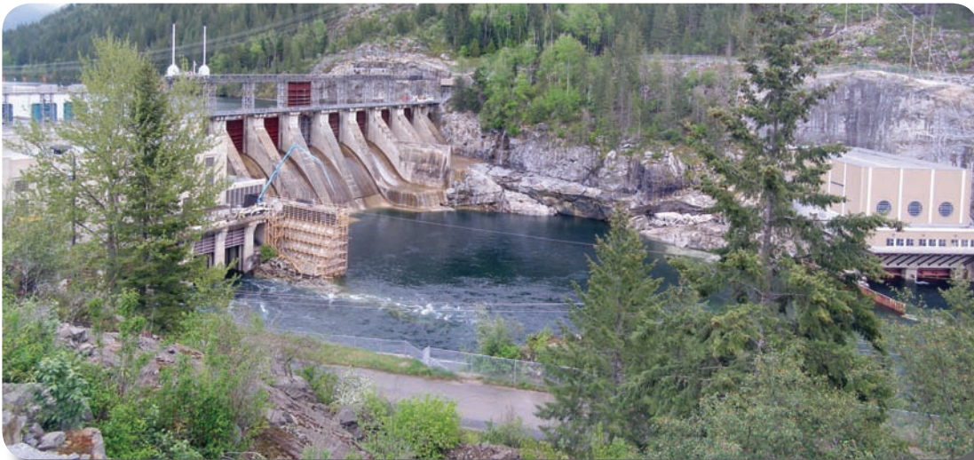
Concrete rehabilitation work began on the Brilliant dam in the spring of 2010. The Brilliant Expansion Generating Station is located immediately downstream of the dam. - Les Stanchuck photo.
