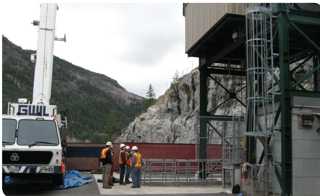
Workers prepare for the intake gate emergency close test that was successfully completed at the Brilliant Expansion in spring 2010.
