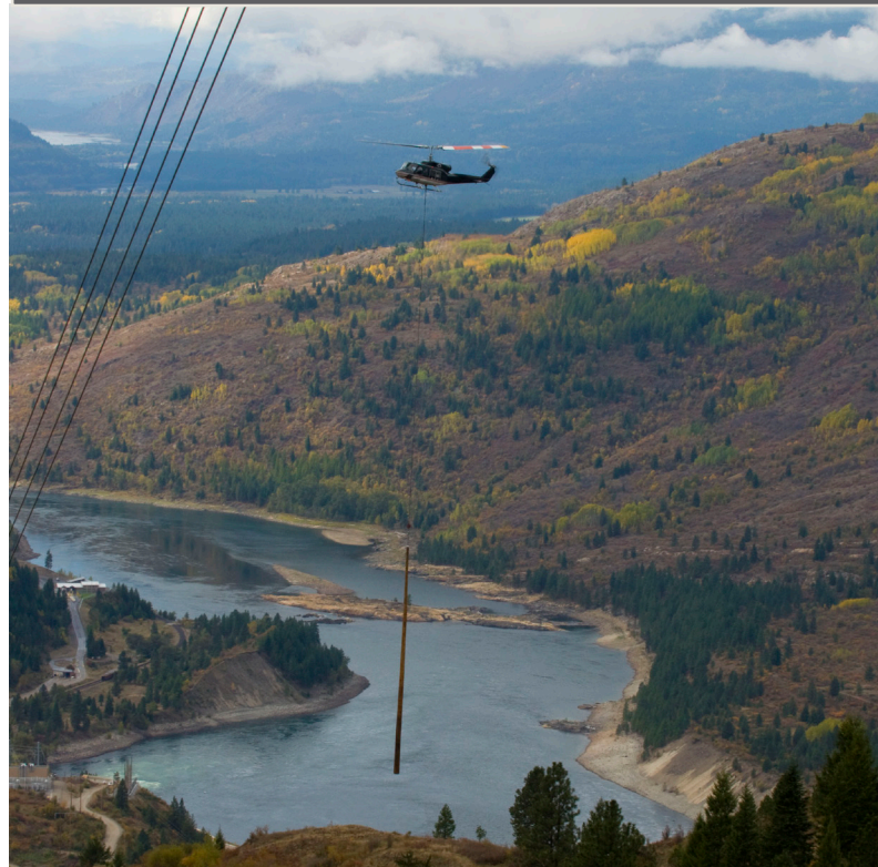
A helicopter placing poles for the new Waneta Expansion 230kV transmission line
