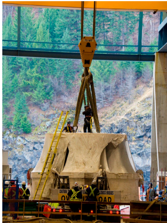
One of the two turbine runners being installed at the Waneta Expansion Project
