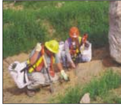
Tree planting taking place along the transmission line for Arrow Lakes Generating Station
